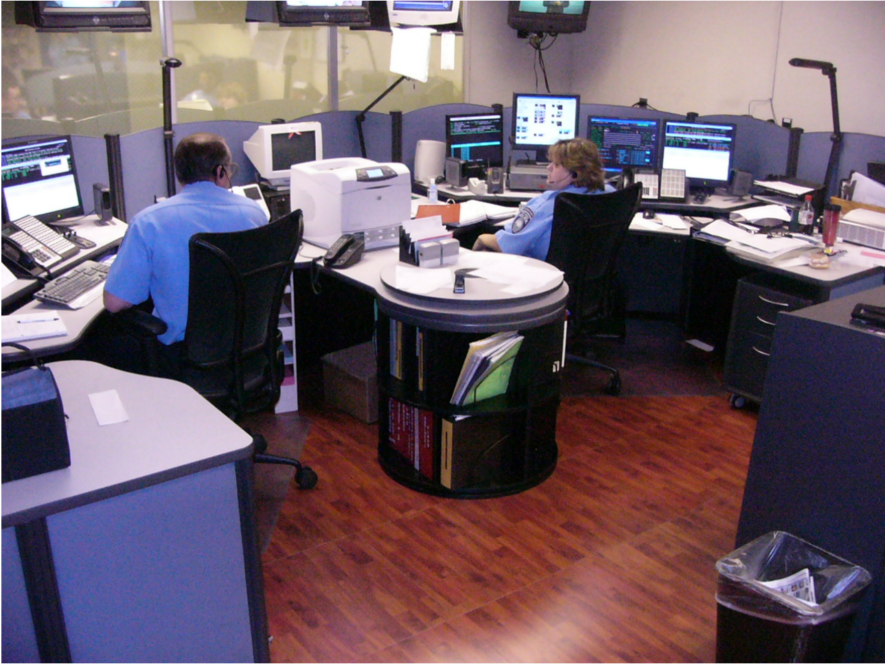
Tech Floor raised floor with Alder Laminate surface finish at Port Huron P.D.
