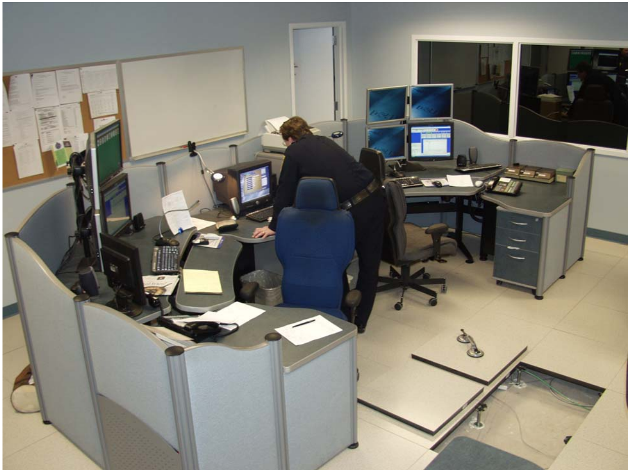
Tech Floor raised floor with Watson Synergy Consoles in Parsippany PD's new Dispatch Center
