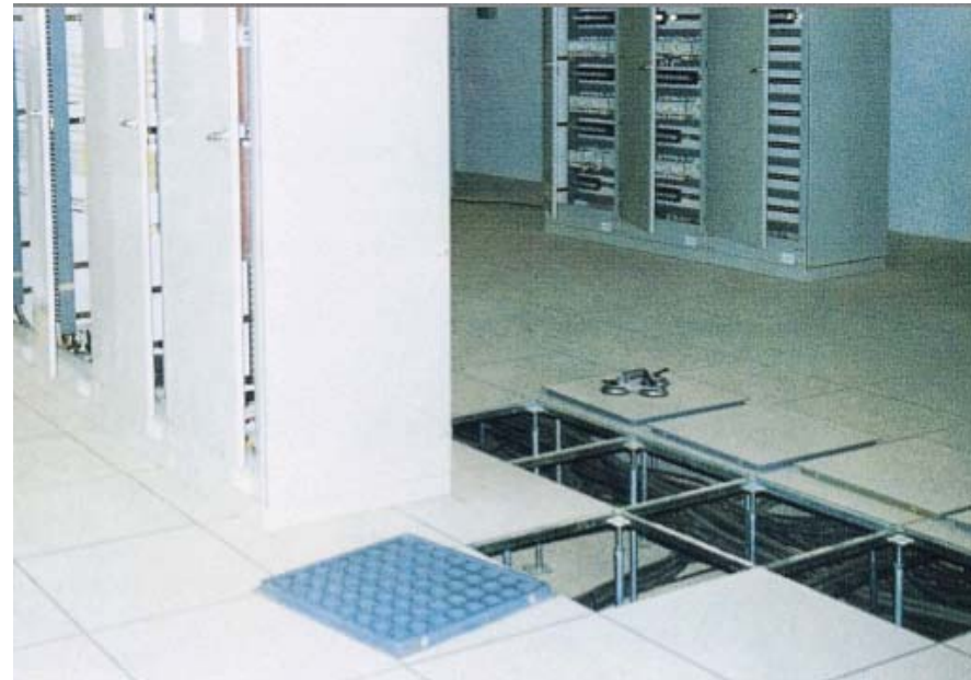
Picture shows a traditional raised floor
